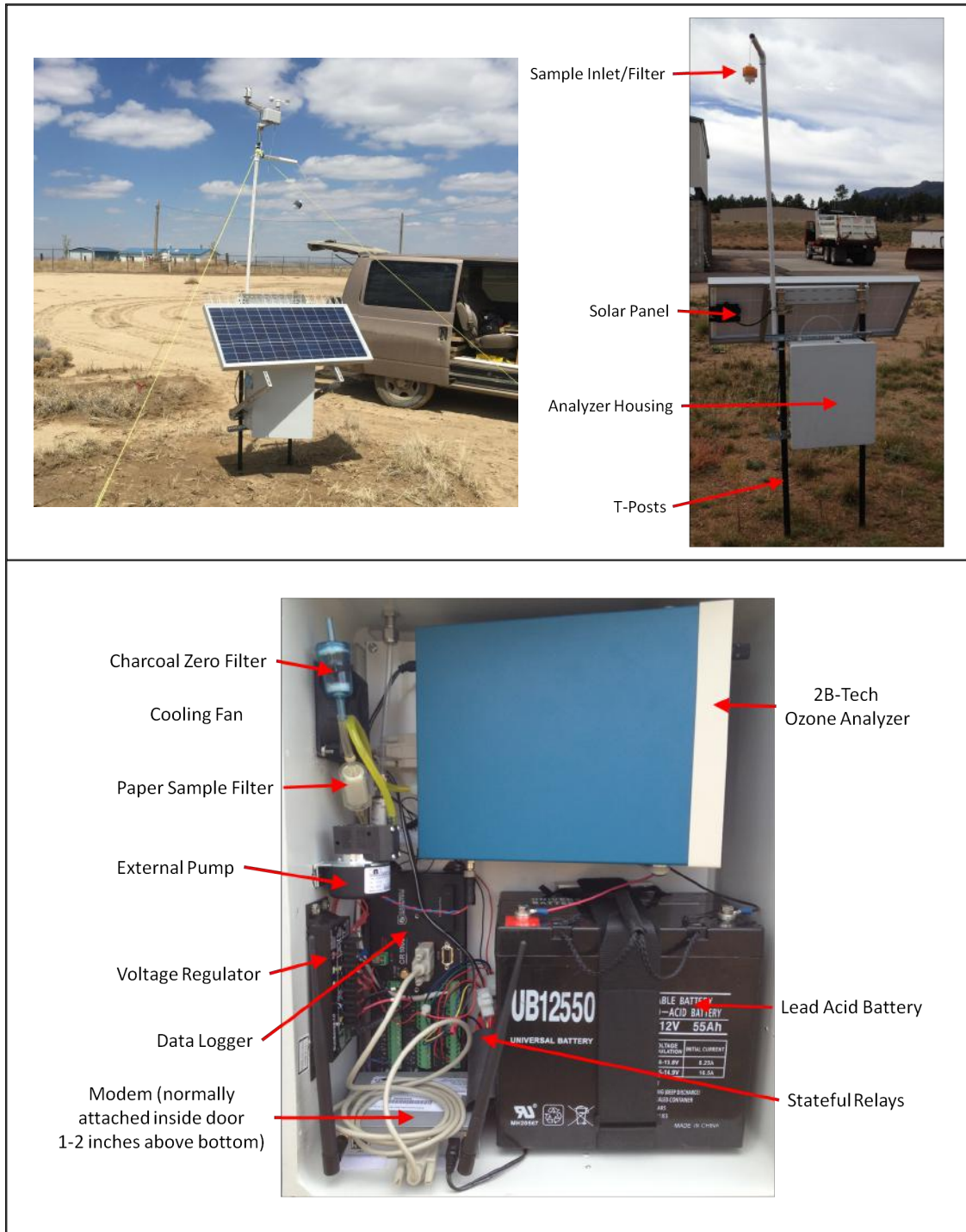
Figure 1.4: Top left: APCD monitoring equipment at the Huerfano site, including a solar-powered ozone monitor and met tower. Top right: Schematic of the monitoring system showing the location of the sampling inlet and instrument shelter. Bottom: Detailed schematic of the instrument shelter showing the location of the 2B Tech instrument, battery, data logger, and other miscellaneous features.
